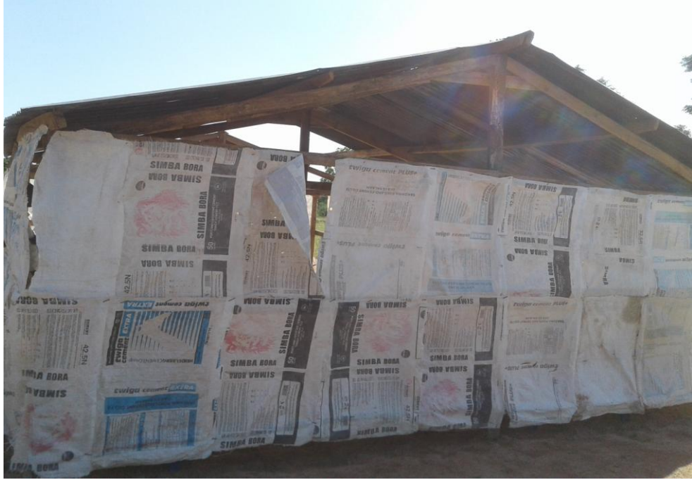
THIS IS A NEW BRANCH IN MWANZA THEY NEED $ 1380 TO PURCHASE THE LAND, THEY ARE RENTING AT PRESENT BUT PLANS IS TO PURCHASE THE LAND AND START CONSTRUCTION
